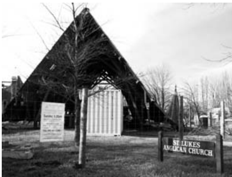
St. Luke's Anglican Church in Christchurch, which was badly hit by the earthquake.
